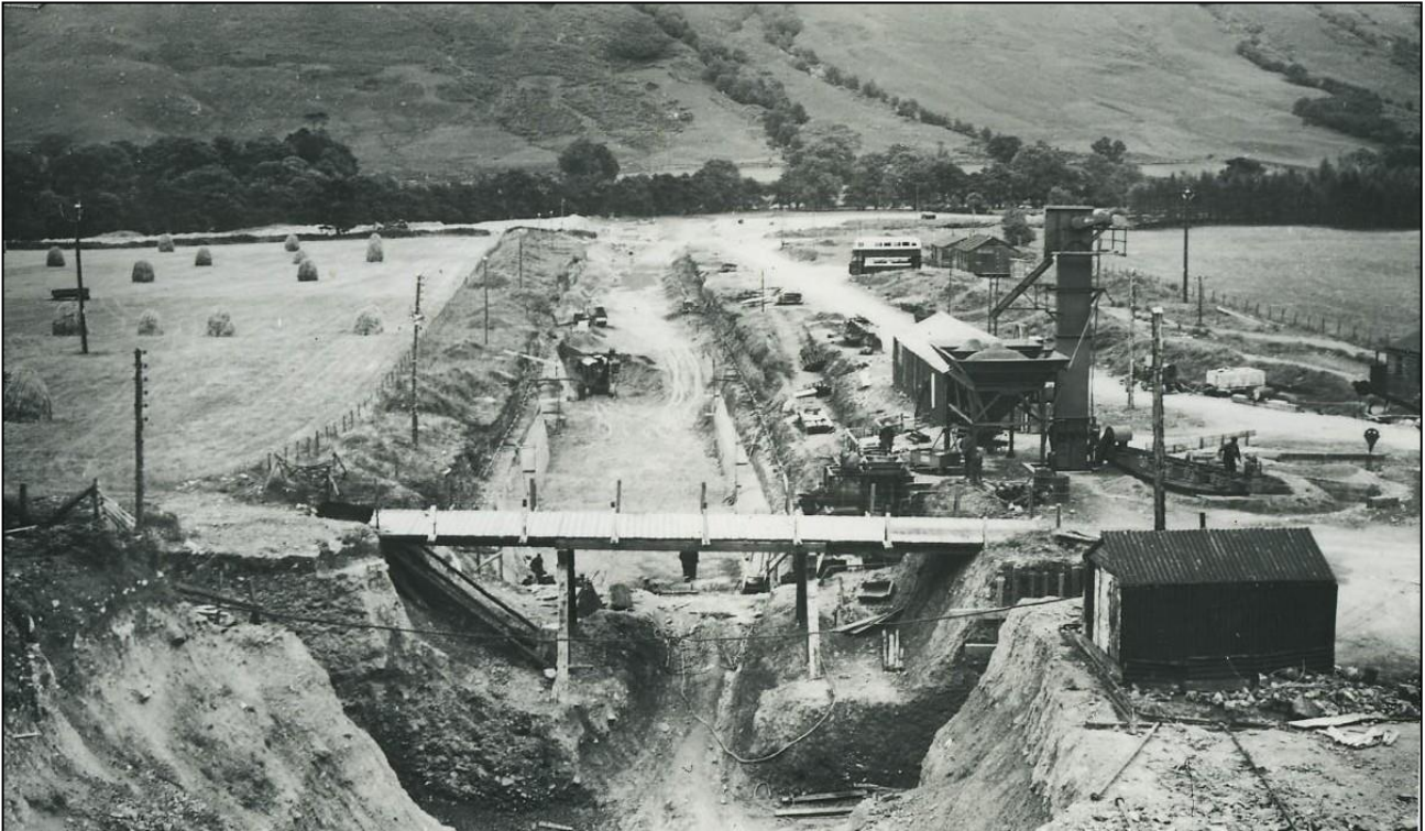
View of Tail Race Clachan Hydro Electric Scheme 1955
